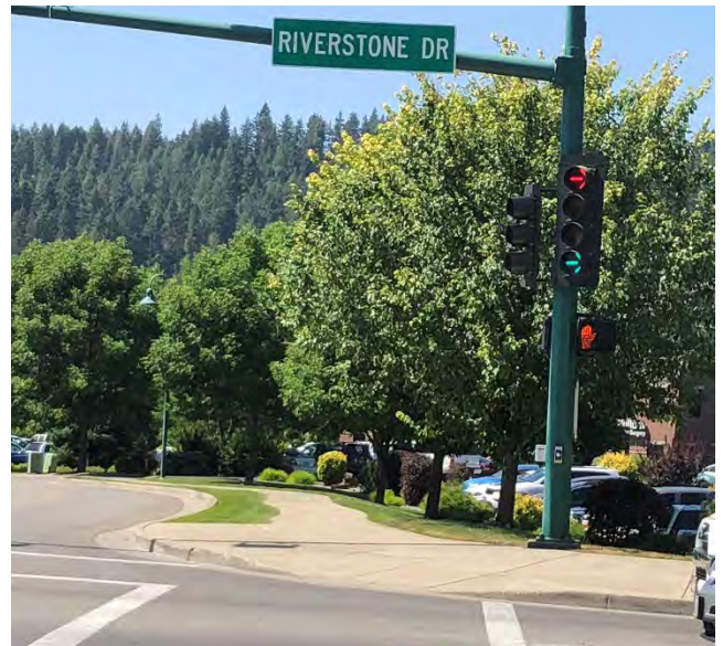
Figure 7-4: Signal head malfunction at Riverstone/Lakewood
